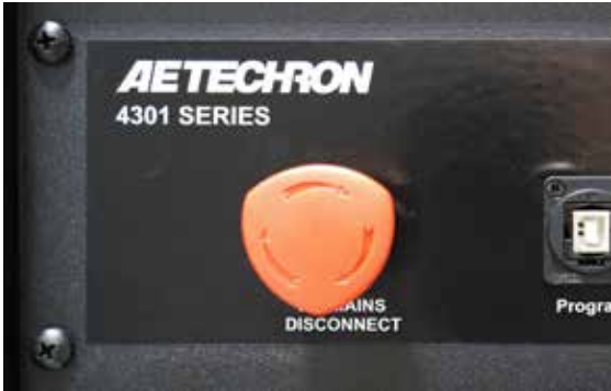
Figure 3.1 – AC Mains Disconnect Switch
